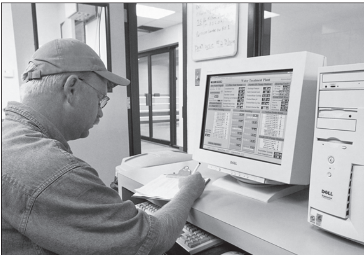
SCADA security systems are vulnerable to hacking and viruses.
