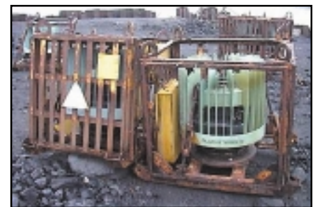
Abandoned Soviet RTGs. The former Soviet Union used RTGs for unmanned lighthouses and navigational beacons. photo credit: Finnmark region government (c) .
